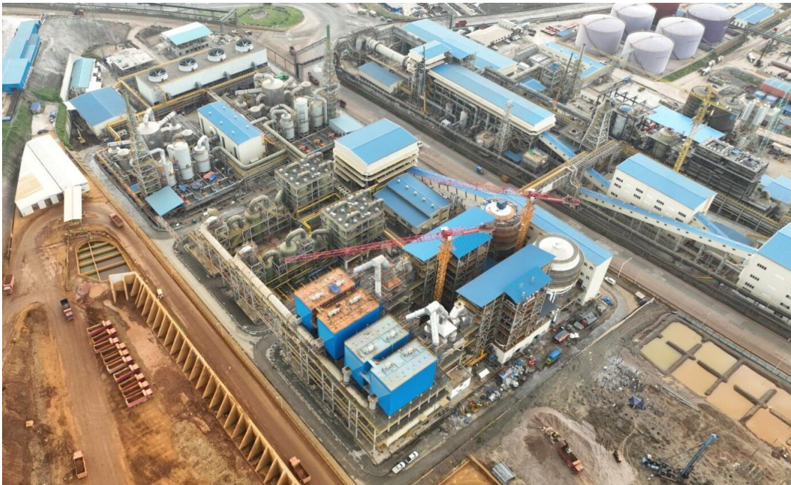
Figure 4: AIM Project acid plant
