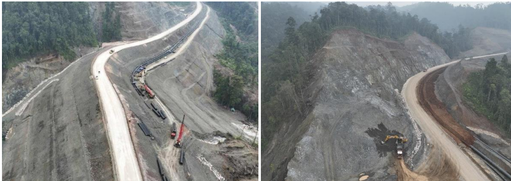
Figure 3: Slurry pipelines construction parallel to hauling roads (left); Hauling roads extension (right)
