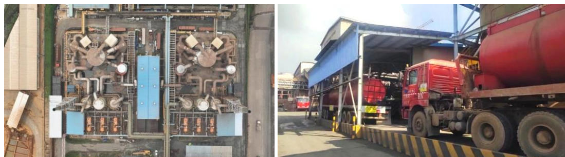
Figure 15: Acid Plant Operation
